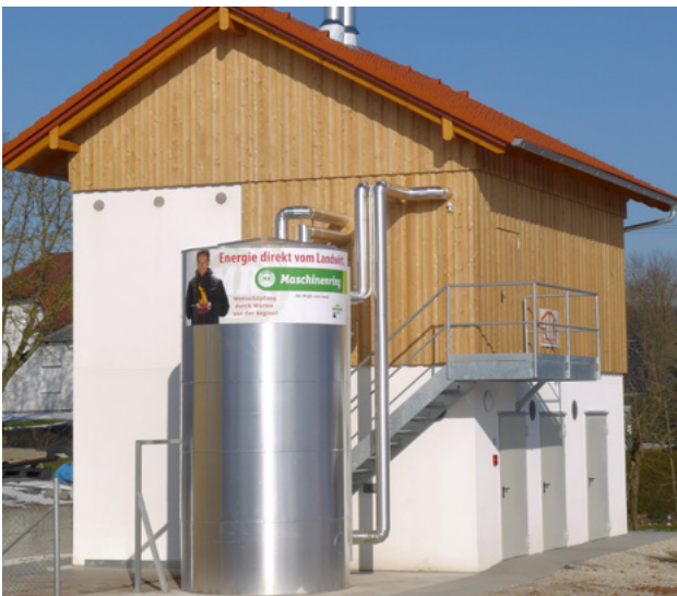
MR Service (Contracting) in Niederthalheim, 550 kW Hackgut
