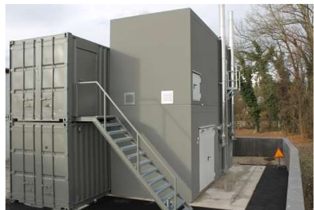
Doppelstock-Heizcontainer 2x90 kW Pellets, Industrie
